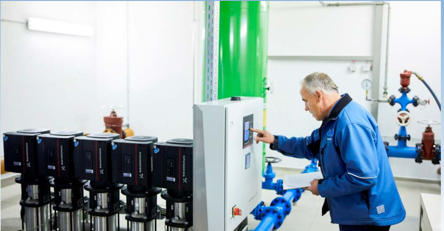
Günter Meisl, chief technician at ZWR, makes his daily rounds at the main pumping station in Wolkertsham with the Grundfos Demand Driven Distribution system CU controller.
