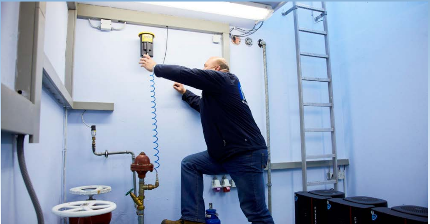
Roland Kainz checks the XiLog pressure sensor at the downstream Opping pumping station. It sends data via GSM to the DDD controller in Wolkertsham.
